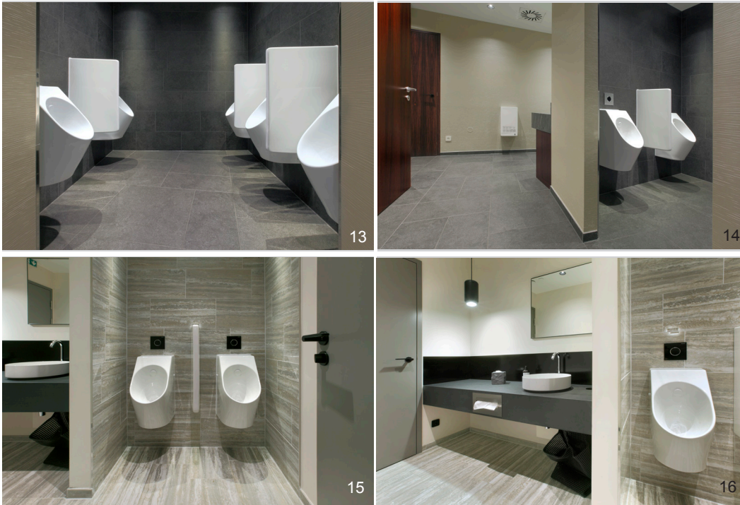
13-16 TOTO urinals are installed in semi-public areas. These rimless urinals are accessible from all sides, making them easy to clean. They feature our CEFIONTECT glaze and moulded odour trap for ideal hygiene. Photo: TOTO
